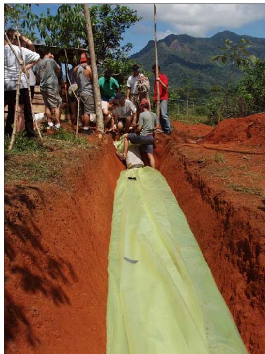
Workshop participants building a micro-scale digester in Costa Rica. Photo by Ian Woofenden.
