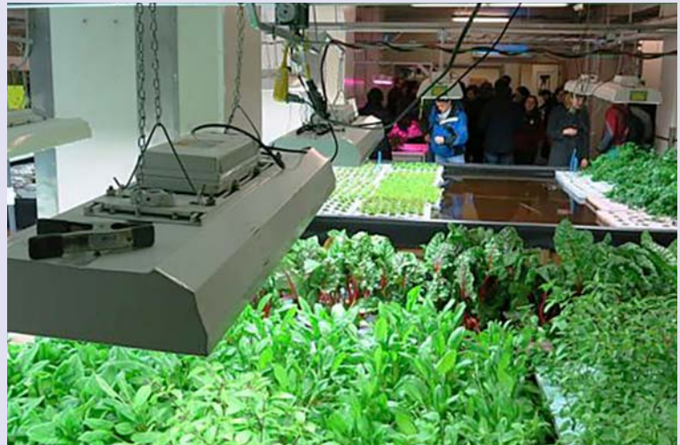
Large banks of fluorescent lamps provide the spectrum of light that keeps the floating beds of plants alive year-round in The Plant Chicago, a vertical farming facility. Source: Peter Gray/Harvest Public Media
